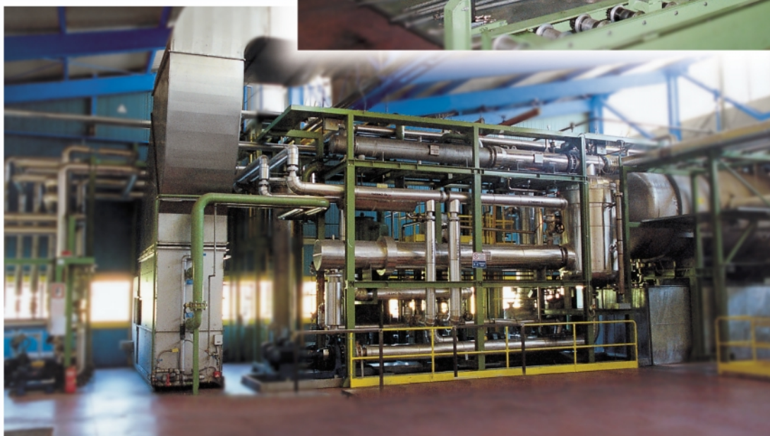
Distillatore e torre evaporativa Distiller and cooling tower
